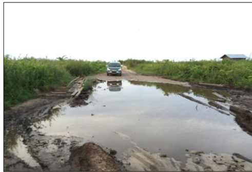
Road Condition of Paloh to districts Paloh
